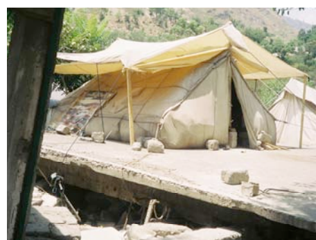
Fig 7: Family camping out on the collapsed roof of their house by the main road in Chella Bandi.
