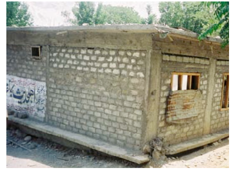
Fig 23: The ground floor of this house in Chella Bandi pancaked, killing the occupants.
