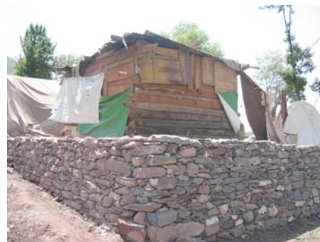
Fig 30: The stone platform has been rebuilt and a temporary shack built, Balakot.
