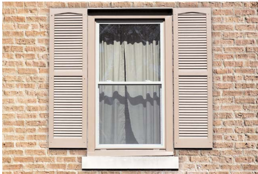
External shutters can be used to mitigate summer overheating
